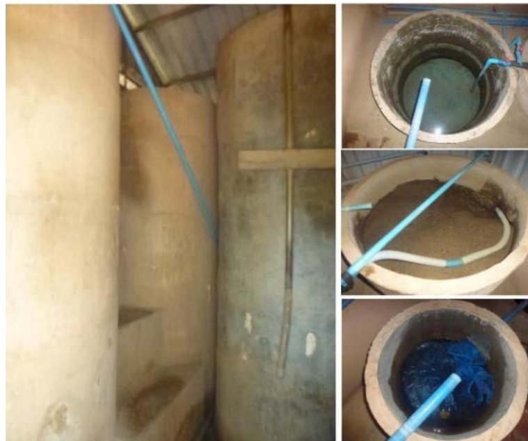
Figure 2. Water storage, percolation, sand filtration and activated carbon treatment at an O-We Water refill kiosk.
