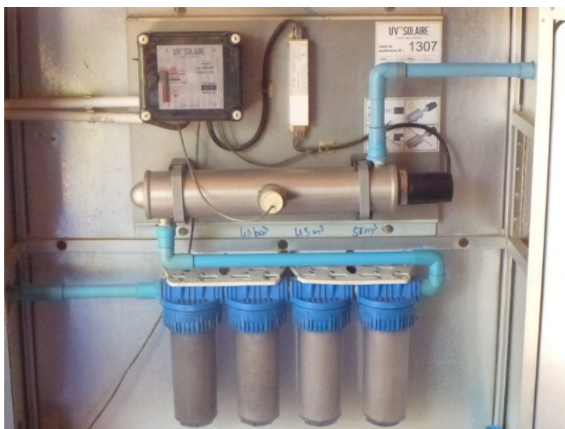
Figure 3. Water filtration and ultraviolet treatment.
