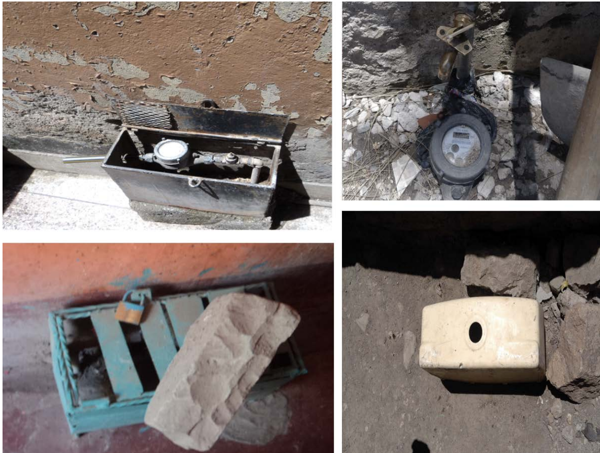
Figure 2. Reassembled metre installations. Clockwise, from top left: a caged water metre; a metre virtually buried in the ground; a metre hidden beneath a repurposed plastic container; and a caged and locked metre, further protected with a heavy stone on top.
