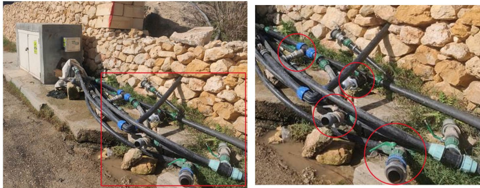
Figure 5. T-valve junctions at the heliport dispenser
