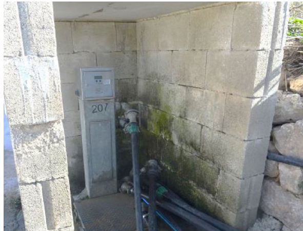
Figure 4. Ghajnsielem dispenser with tylene hose connected
