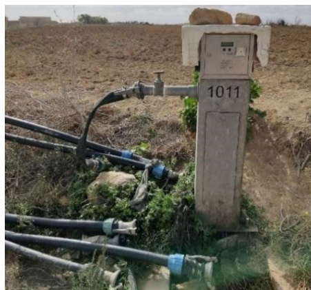
Figure 7. Ghar Ilma dispenser with hoses lying around
