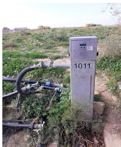
Figure 2. Dispenser with a card reader box on top, a tap on the left side, and hoses that are waiting to be connected
